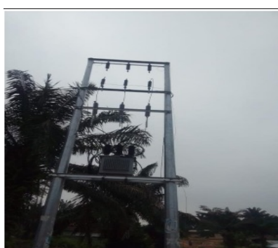
Installed Pole Mounted Transformer
